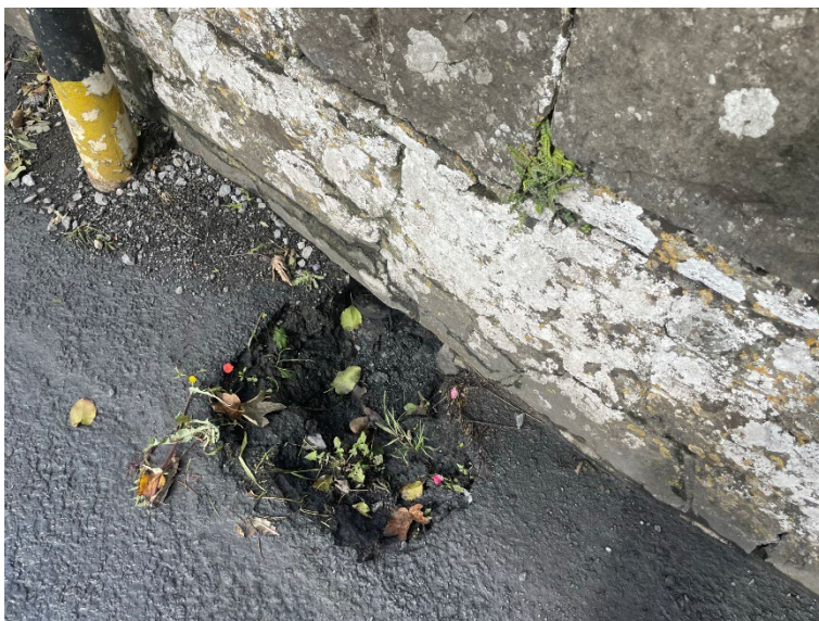
Figure 20 Damaged road surface.
