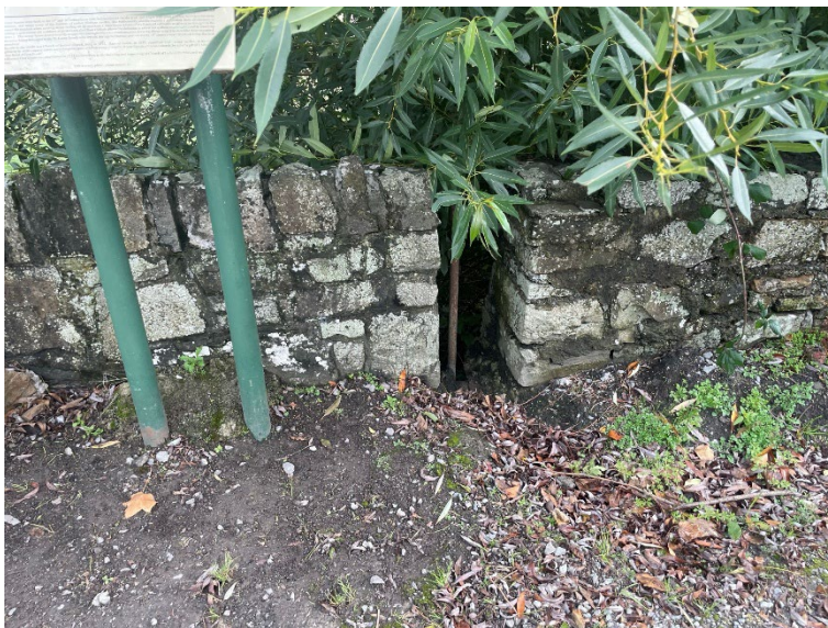
Figure 17 Gap in Parapet where bridge ends, masonry wall continuing along road.
