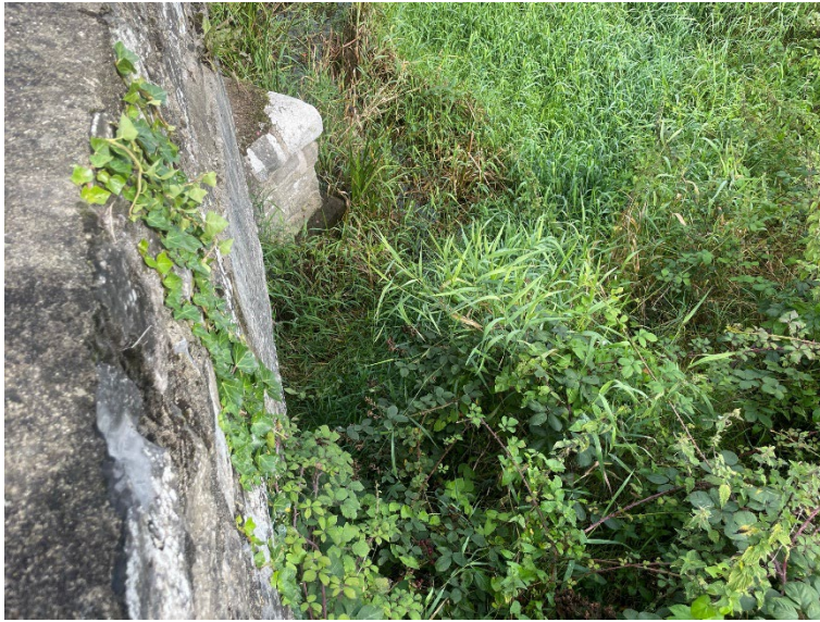
Figure 12 Concrete Capping to Cutwater. Common condition to all upstream cutwaters.
