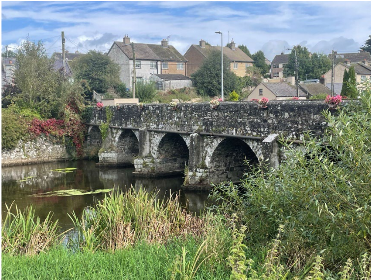
Figure 19 Downstream Elevation with cast iron watermain along elevation supported by concrete columns above masonry cutwater. Vegetation growth along elevation.
