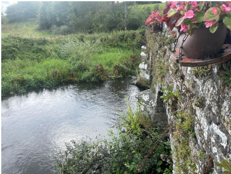
Figure 13 Upstream Cutwaters CW-01 to CW 04. Upstream Elevation with vegetation growth.
