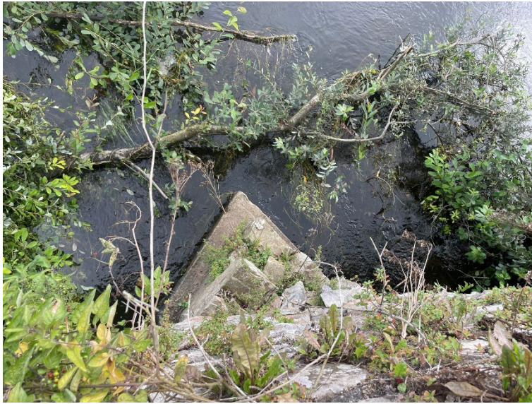
Figure 15 Damaged Cutwater 05 [CW-05]
